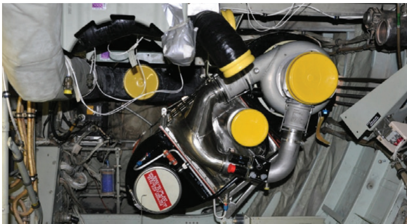
New ECS Refrigeration Unit
